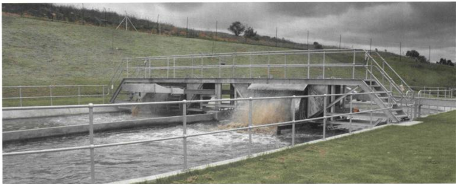
Tecrover's patented horizontal aerators/pumps, to satisfy oxygen demand in reactor and pump mixed liquor into the secondary settling tank
